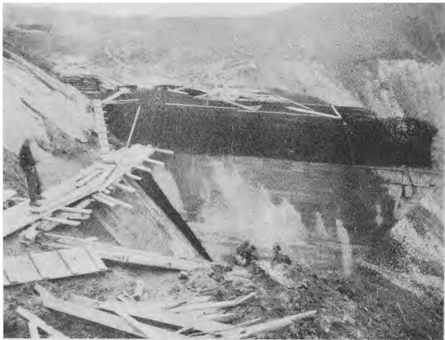
Note damage caused to dome supporting rib by near miss of 12,000 lb. "Tall boy" bomb.
