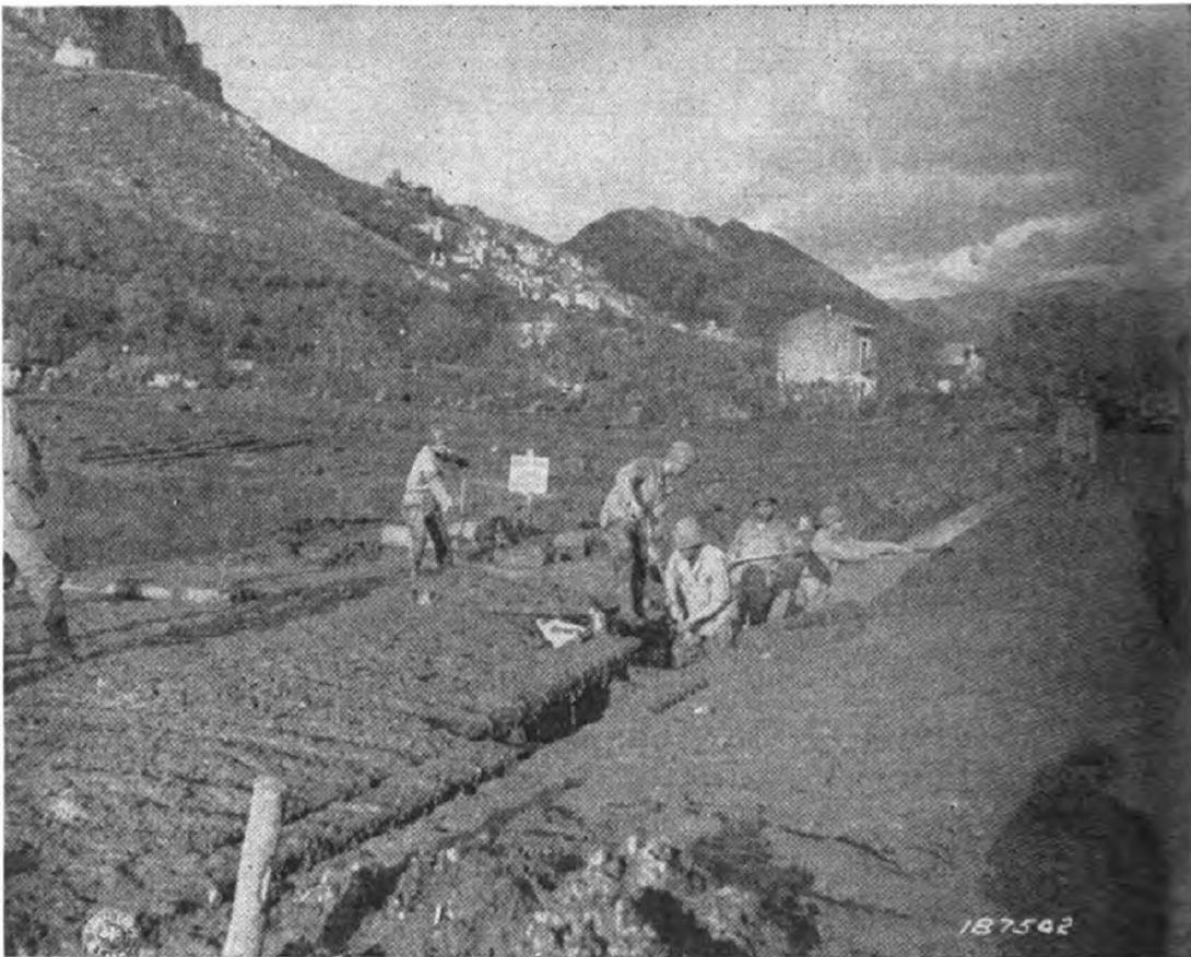
Figure 11. Drainage Canals are Being Built to Drain Off Water in a Field to be Used as an Ammunition Depot, in Italy, Dec. 1, 1943.
