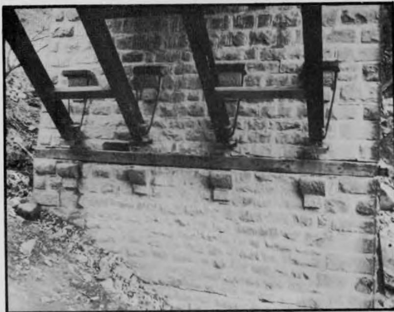
CRACK IN PIER AND WEDGE
