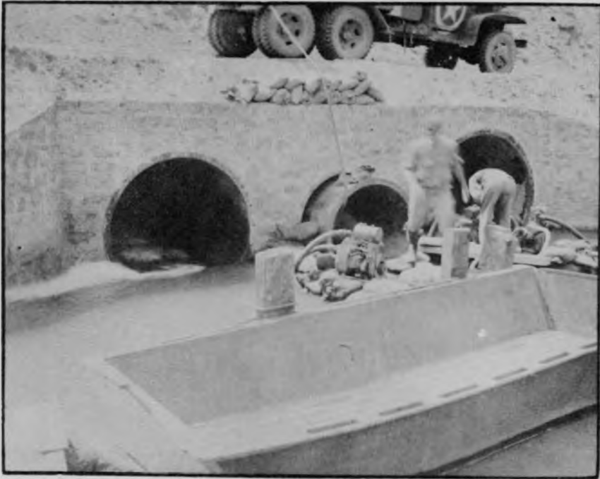
Figure 7 Placing of Inlet Connection to Existing Pipe Culvert by Arcwelding and Grouting.
