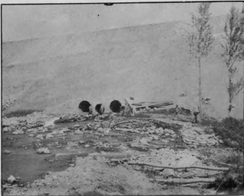
Figure 8 View of Outlet End of Existing Pipe Culvert. Pipe Being Prepared for the Installation of Siphon Con- nection.
